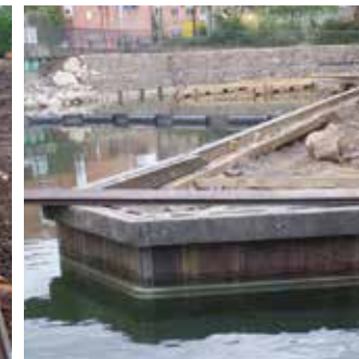
Sheet piling port with rubbing strips
